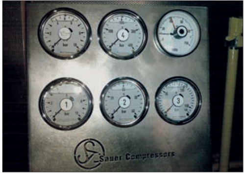
Fig. 33: Compressor monitoring via pressure gauge panel
